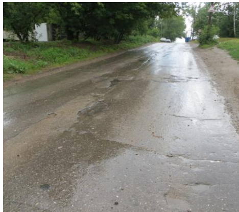
3 Badly worn road
